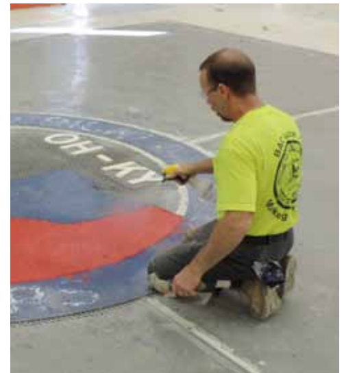
Field Representative Dennis McGraff works on a Terrazzo Ohio-Kentucky Seal at the SORTC.
