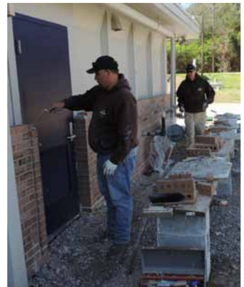
PHOTOS: COURTESY OF LOCAL 8 Field Representatives Shawn Herzog and Keith Hocevar get their trowels out to help renovate the SORTC.
