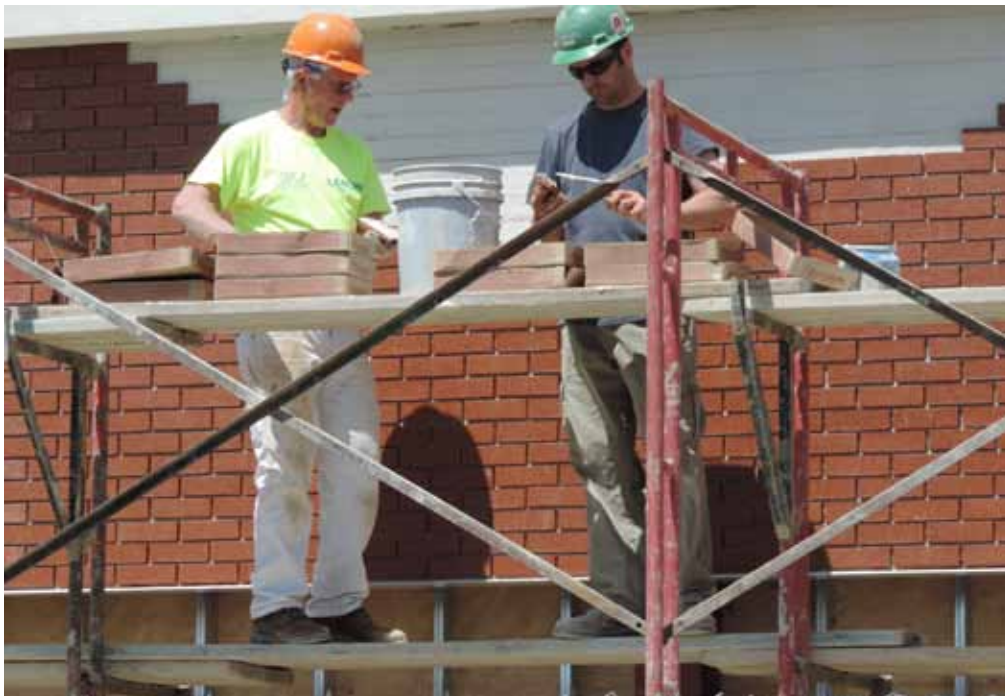
Ljubodrag Andjelkovich of Local 8 and Bryan Linkous of Local 10 install “Thin Brick Veneer” at Tiffany Square Plaza in Boardman.
